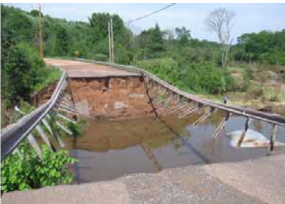
Close to the Pilgrim Community Forest trailhead, the culvert and roadway at the Paradise Road crossing of the Pilgrim River were destroyed.
